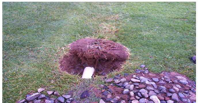
Drain opened up because it is backfilled with soil and ineffective
